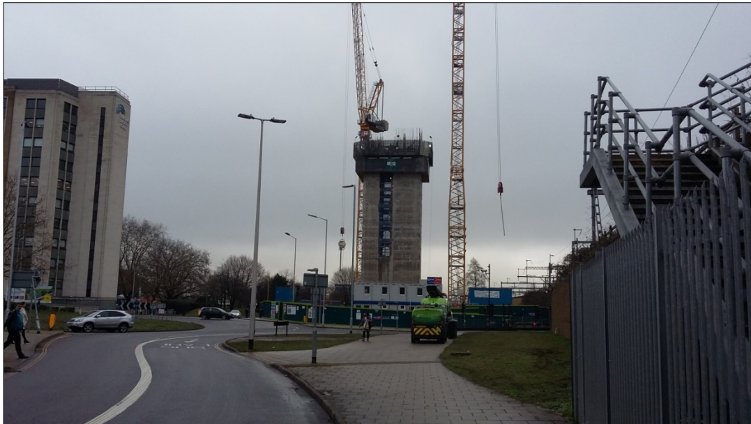
Site photograph looking approximately East from Vastern Road, showing progress on the lift core of permission 162166 (the lift core is now fully constructed to 23 storeys)
